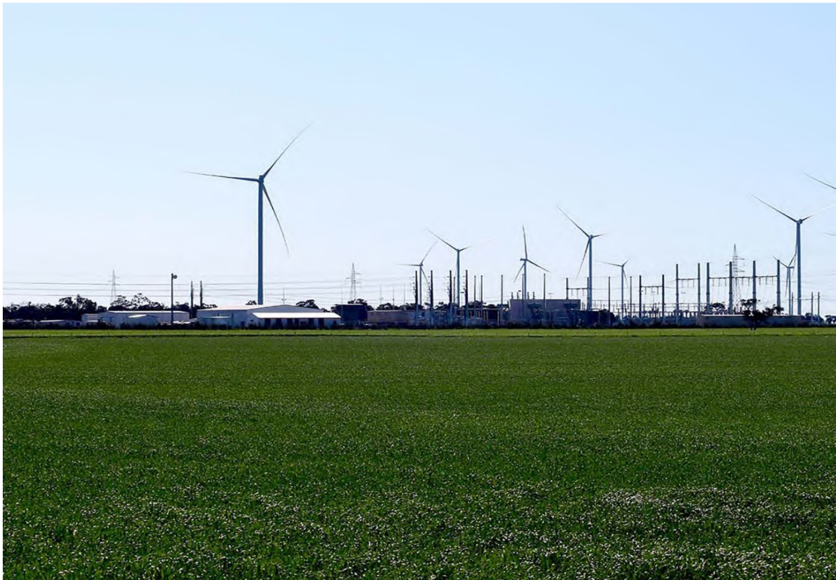
Plate 4 – Main substation and operations centre, Murra Warra Wind Farm, Murra Warra VIC (Image: ©GBD 2022)
