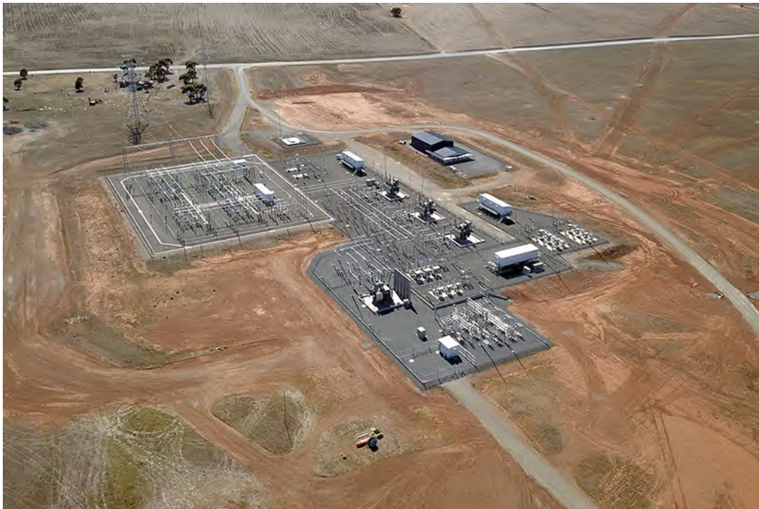
Plate 2 – Typical substation facility, Hornsdale SA (Image: GBD 2018)
